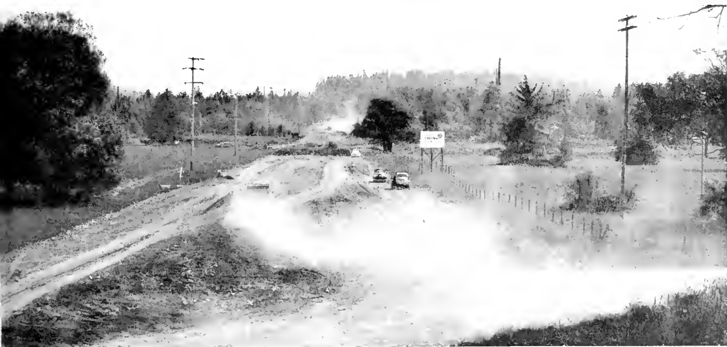
Looking south from the north end of project showing grading in progress on the only portion of alignment which was relatively clear of brush or trees. Clearing here involved only the removal of occasional stumps from approximately 3,000 feet of pasture land.
